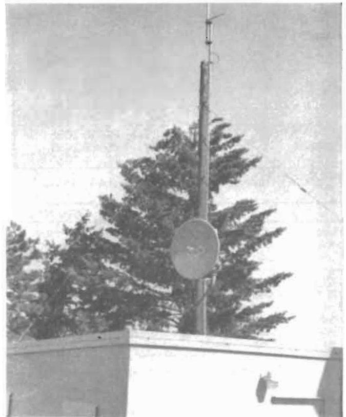
Fig. 4. A simple pole-mounted microwave antenna dish is shown.
